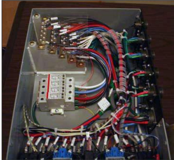
Power Distribution Unit, Interior View
